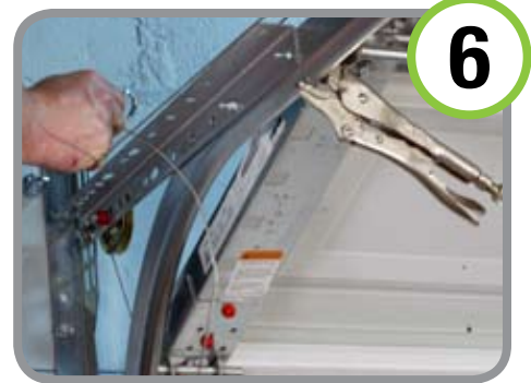
Unhook door cable from it's attachment point at door track near jamb/header
